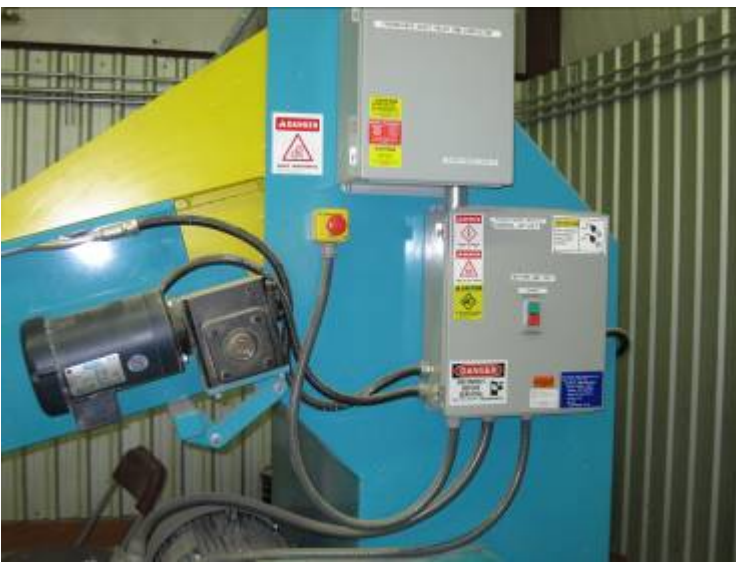
Image 8.2.2: Conveyor and Grinder Electrical Panels
