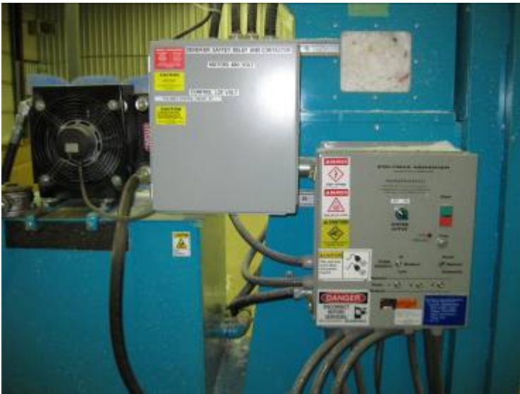
Image 8.2.4: Denisfier Electrical Panel
