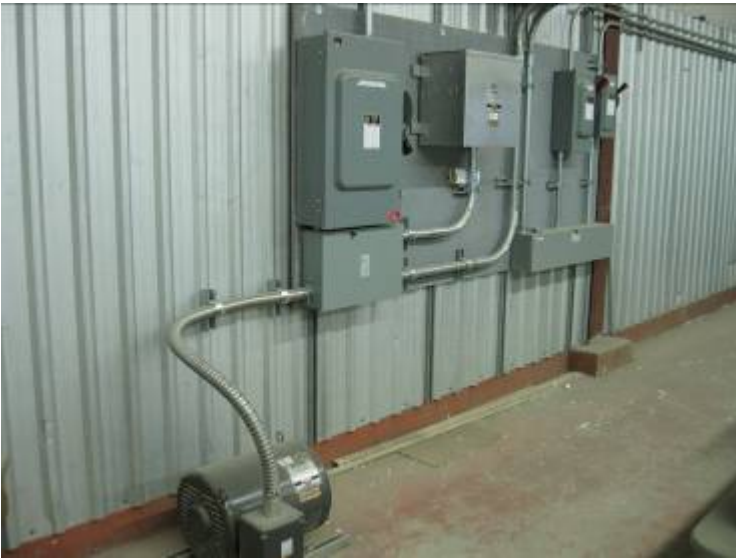
Image 8.2.1: Electrical Panel and Transformer
