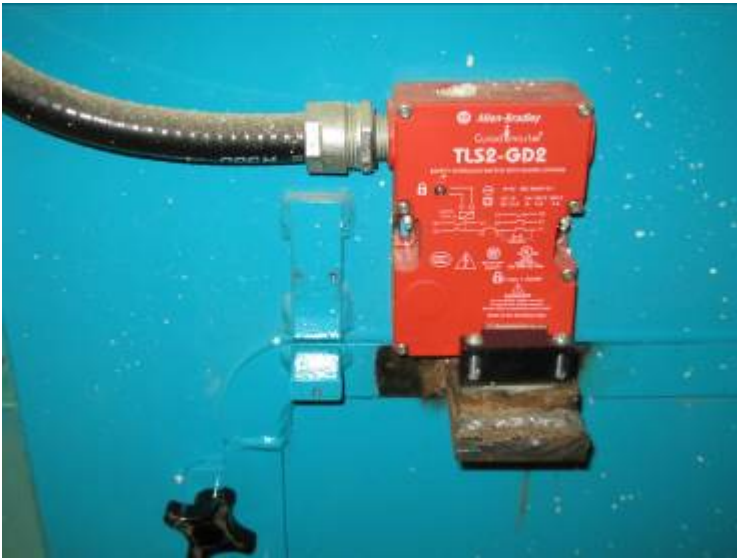
Image 8.2.3: Safety Lockout Switch on Grinder
